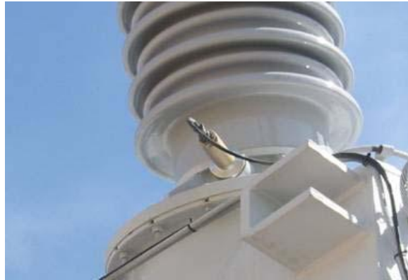
Figure 4: Sensor Attached to the Bushing
