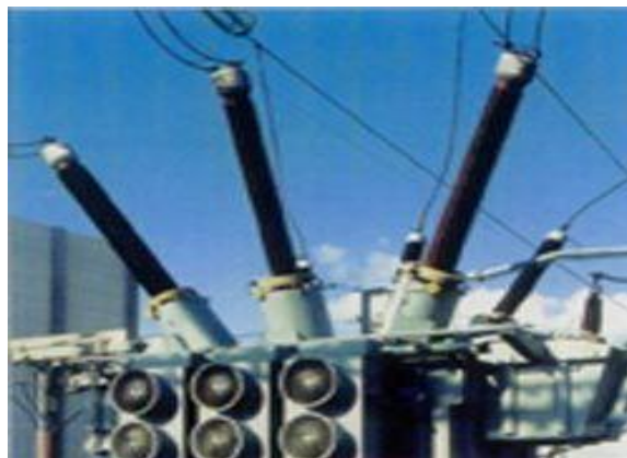
Figure 3: Transformer with Bushing
